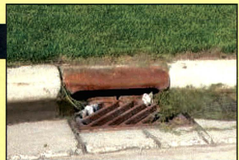
Stormwater Inlet (Courtesy of http://www.grandforksgov.com/government/engineering/land-development/stormwater-information )
