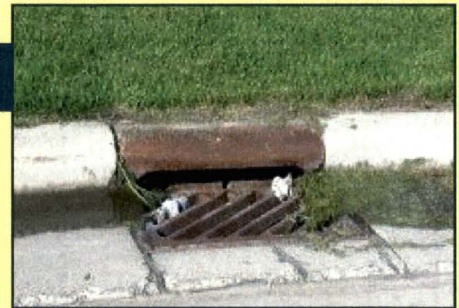
Stormwater Inlet (Courtesy of http://www.grandforksgov.com/government/engineering/land-development/stormwater-information )
