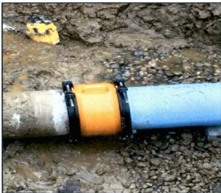
Connection of Rugby's new and old water main (Courtesy of Interstate Engineering)
