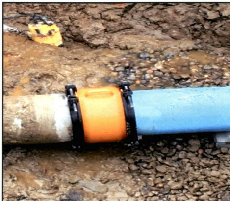
Connection of Rugby's new and old water main (Courtesy of Interstate Engineering)
