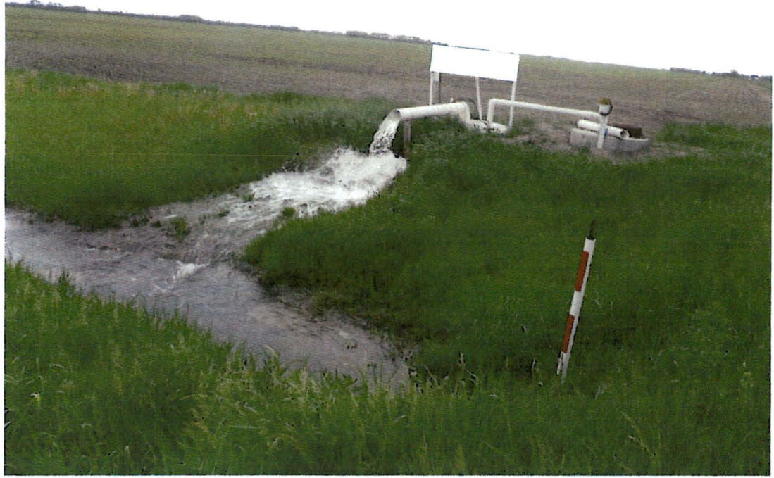
Drainage pump station discharge mixes with surface runoff.
