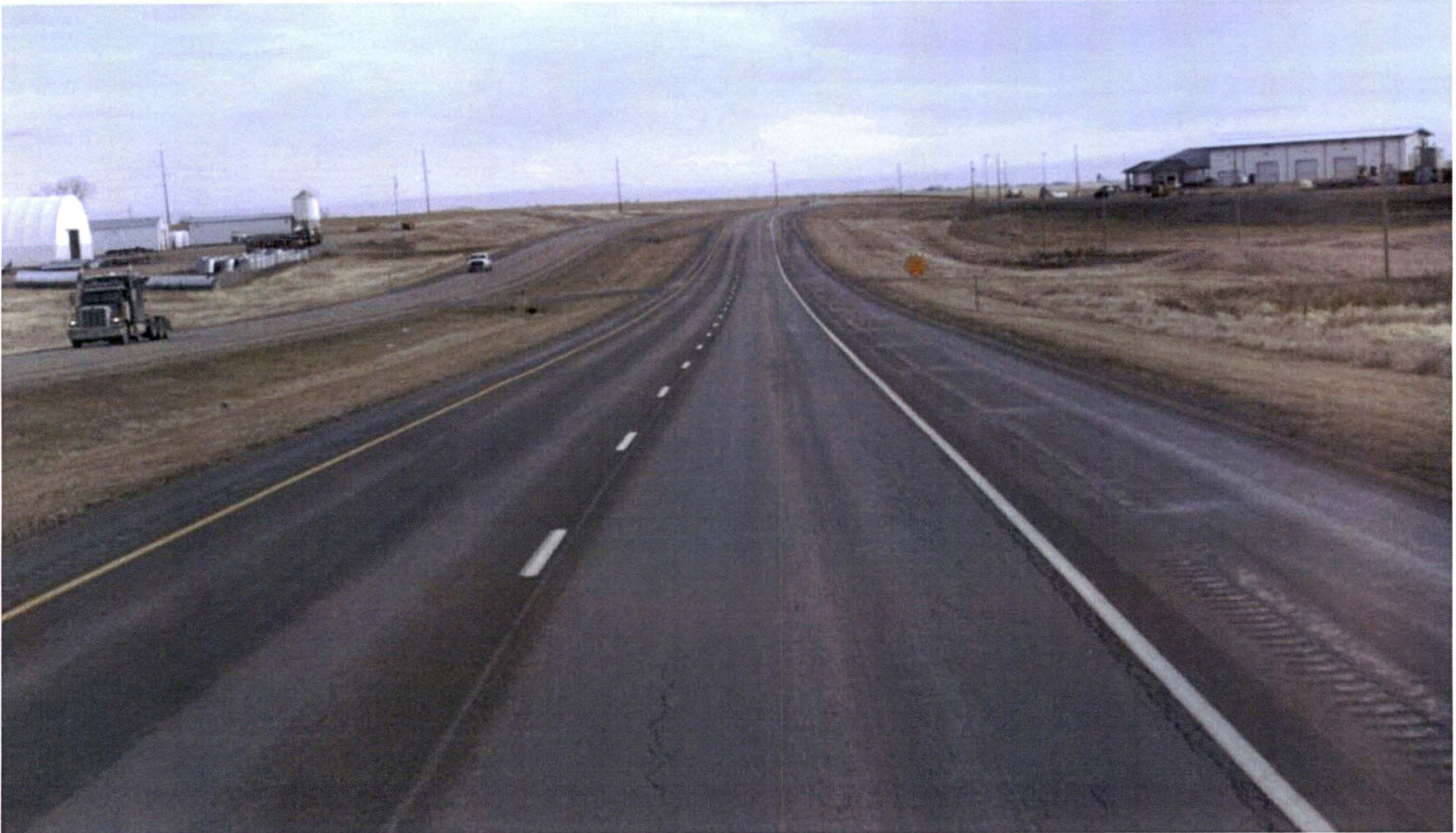
Rutting on US Highway 2 Eastbound from Stanley to Palermo.
