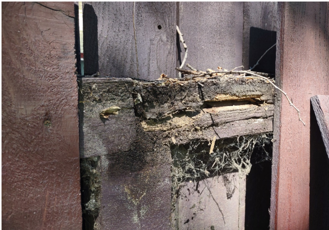
Former Governors' Mansion - Exiting Fence Wood Rotting
